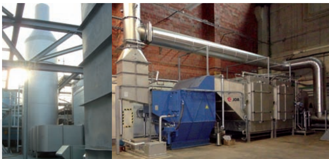
Structured Packing tower / 3-Stage Odor abatement unit including the JOA inline-venturi™ scrubber (low energy usage)
