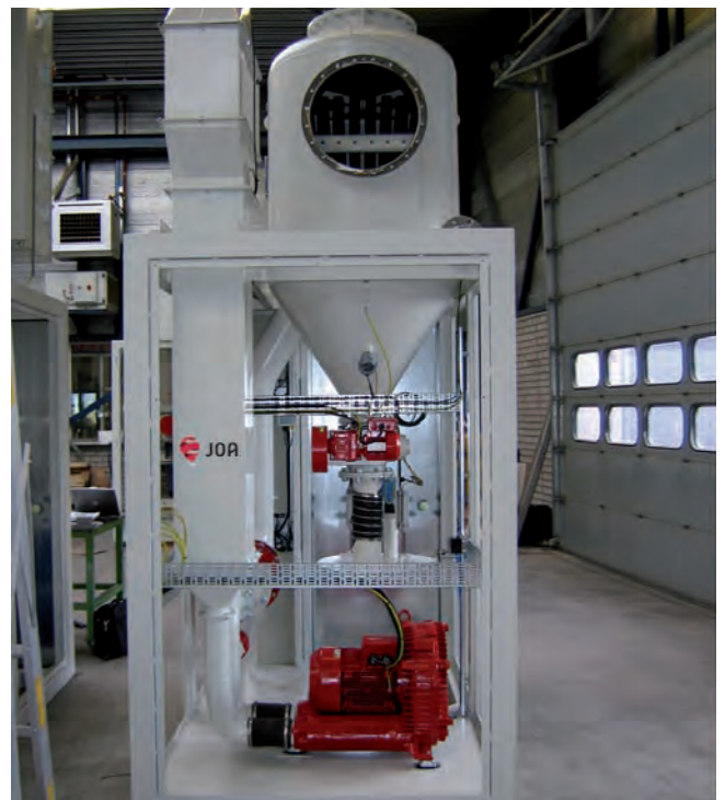
Centralized explosion safe CVC units handling housekeeping of toner production lines.
