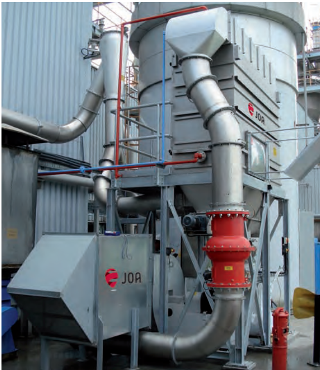
Explosion safe dust collector for plastic compounding operation.
