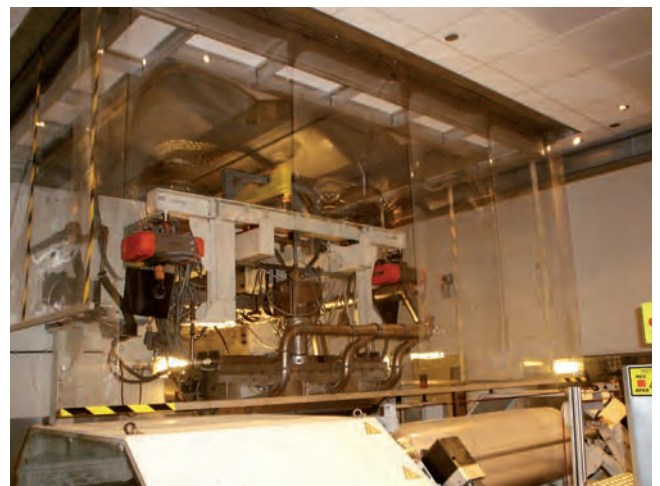
Clean room ISO class 6, with Microclimate™ technology for eliminating the 'thermal engine'.
