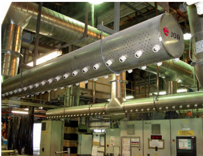
Effective JOA evaporative cooling combined with Cooljet™ distribution in the target areas.
